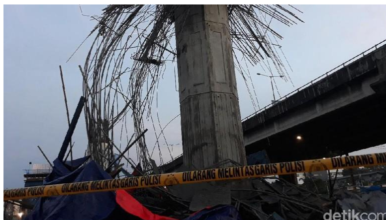
Tiang girder Tol Becakayu ambruk (Foto: Tsarina Maharani)
